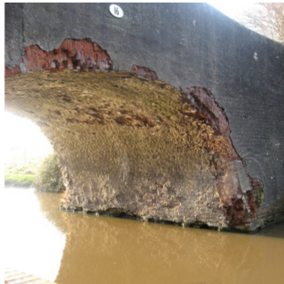
The early brick bridges show considerable dilapidation.
