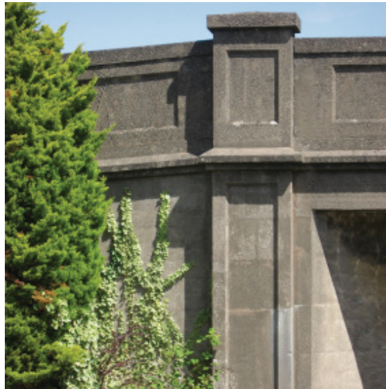
Concrete road bridge - Bilford Road - designed with elegance and still weathering well.
