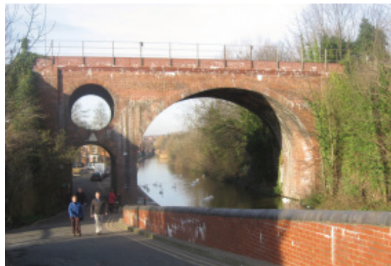
Railway viaduct - a feature of special significance and on the council's 'local list'.
