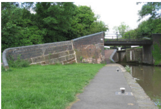
Bridge No.13 has an iron span from early in the 19th century.
