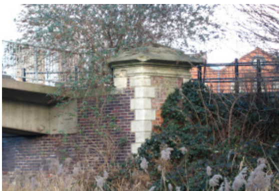
One of the surviving piers to the old bridge at Cromwell Street.
