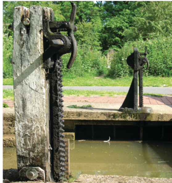
Wooden post supporting side paddle gear, and new type steel replacement, Lock 5
