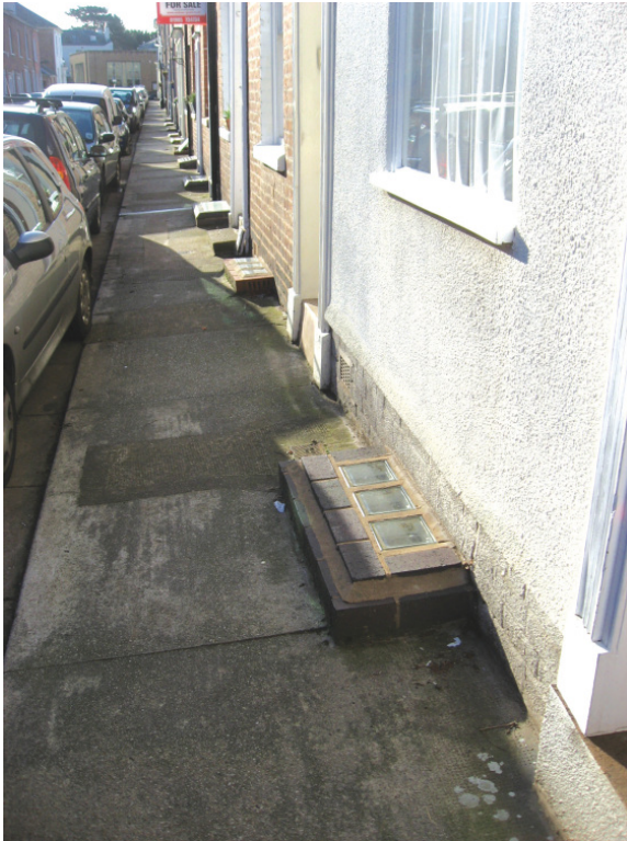
Poor concrete pavement surface - York Place
