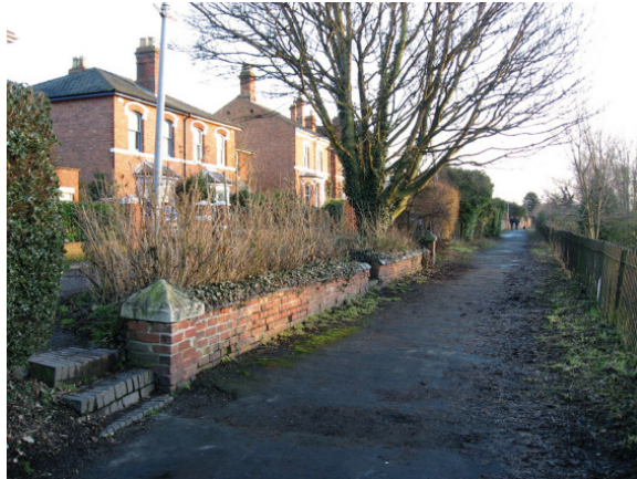
Problems with significant retaining wall.
