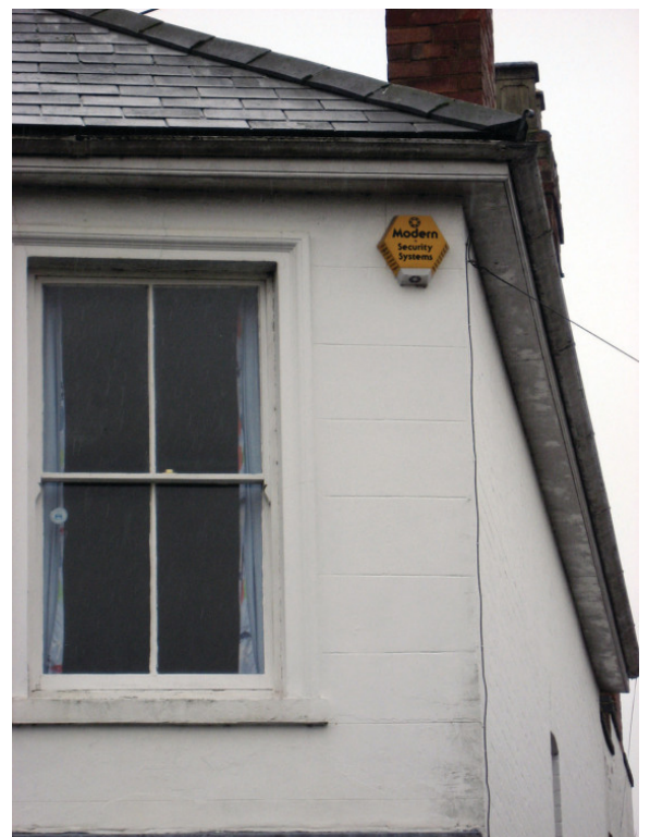
Unfortunate modern addition - security alarm.
