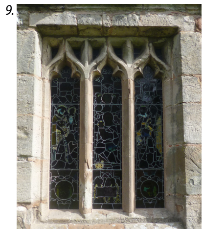
7. Cast iron gatepost, churchyard 8. Sash windows, Church House 9. Stone tracery window, Claines Church
