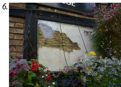
4. Door Case, Church Institute 5. Mock timber-framing, Church Institute 6. Retained wattle and daub infill panel, Mug House
